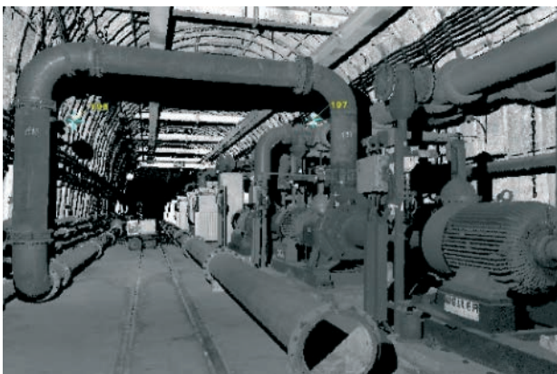
Point cloud of a pumping station
